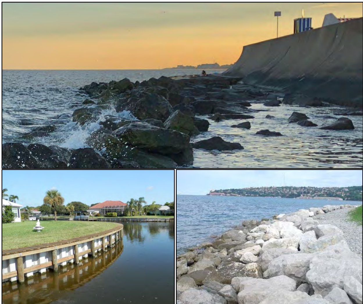
Fig. V.A.1. (a) A seawall in Galveston, Texas; (b) Bulkheads in Florida; (c) Rock armor revetment on the coastline between Lucija and Seča (Source: https://www.galvestonunscripted.com/seawall-galveston-texas ; https://www.eastcoastdocks.com/seawalls/ ; https://www.researchgate.net/figure/Rock-armor-revetment-coastline-between-Lucija-and-Seča_fig1_335930897 )
