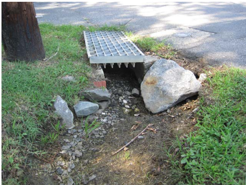
Photo of Inlet at Caroline Street and Morris Street (Photo taken by GMB)
