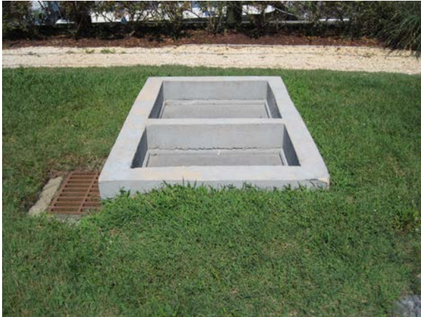
Tide Gate Vault at Banks Street Outfall (Photo taken by GMB)
