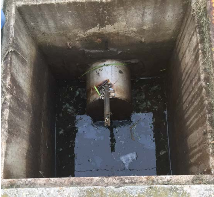
Causeway Tide Gate (Photo by GMB)
