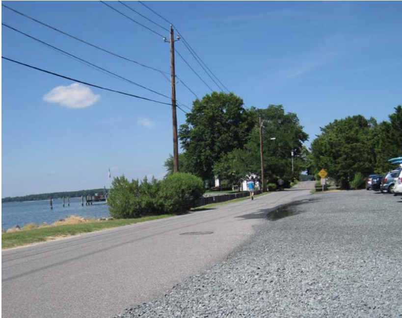
Ponding area along The Strand at Town Parking Lot (Photo by GMB)
