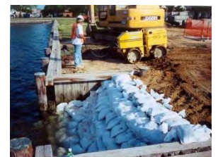
Elimination of "duckwalk" to solve flooding issues on Water Street, Cambridge, MD
